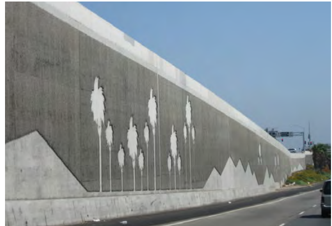
Sound walls help reduce movement of air pollutants and noise emanating from freeway
